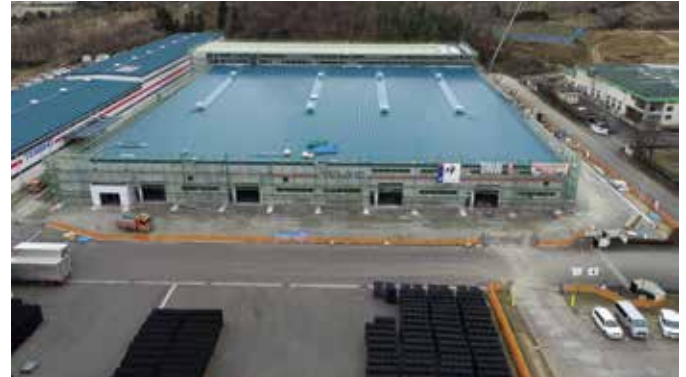
Tensho Electric Industries new Yabuki plant.
